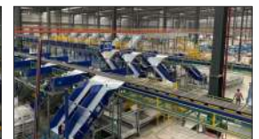
Outfeed / Exit Chutes
